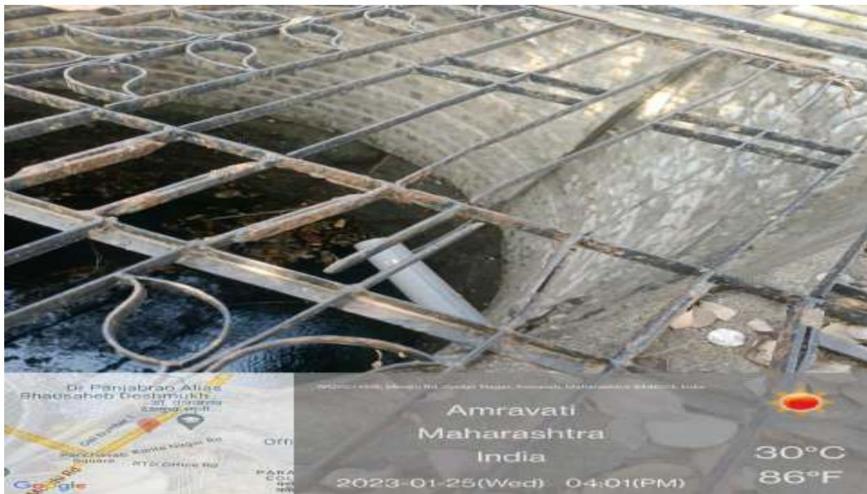
Image 1 Rain water harvesting and filtration setup
